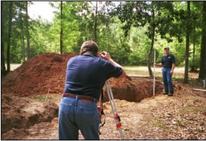
A LASER LEVEL is used to ensure the excavation is level before installing tanks.
