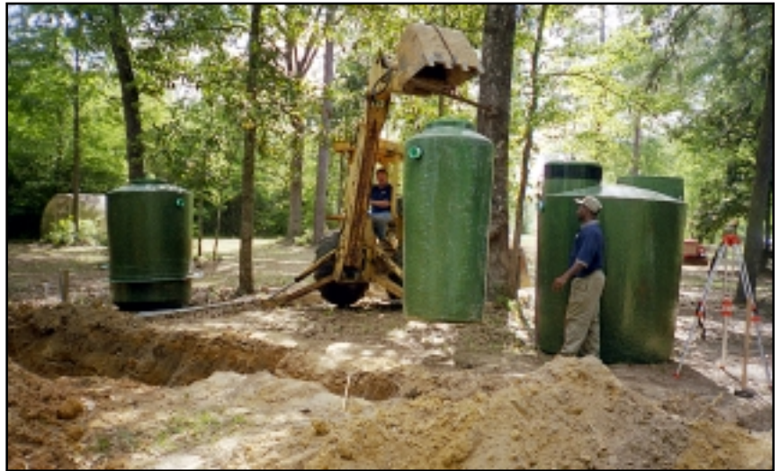
A PRETREATMENT TANK is lowered during installation of an aerobic septic system. The main treatment tank is at right.
