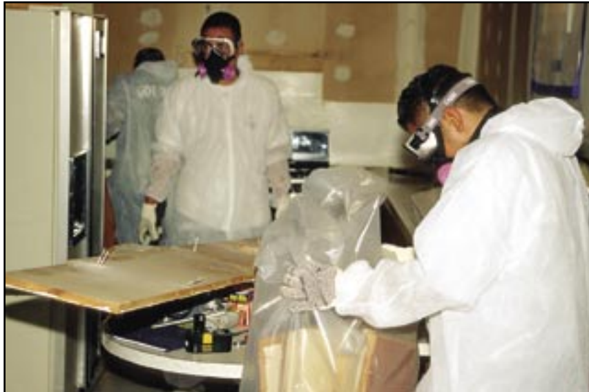
COMMERCIAL REMEDIATION teams follow protocols to remove extensive mold infestations. Most outbreaks can be cleaned using bleach and water.
