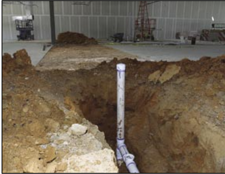
"LEAVE OUTS" IN FOUNDATIONS at Corporate Centre Kirby accommodate the added plumbing medical offices need.
